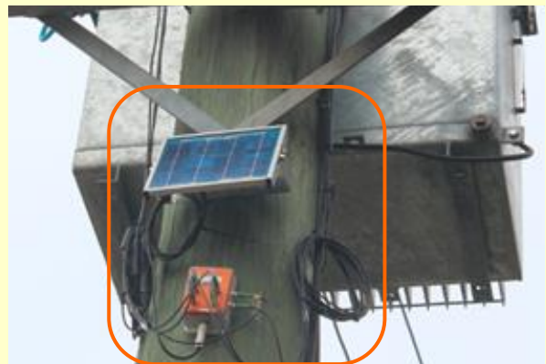
Figure 2: Installation on a pole-top transformer
