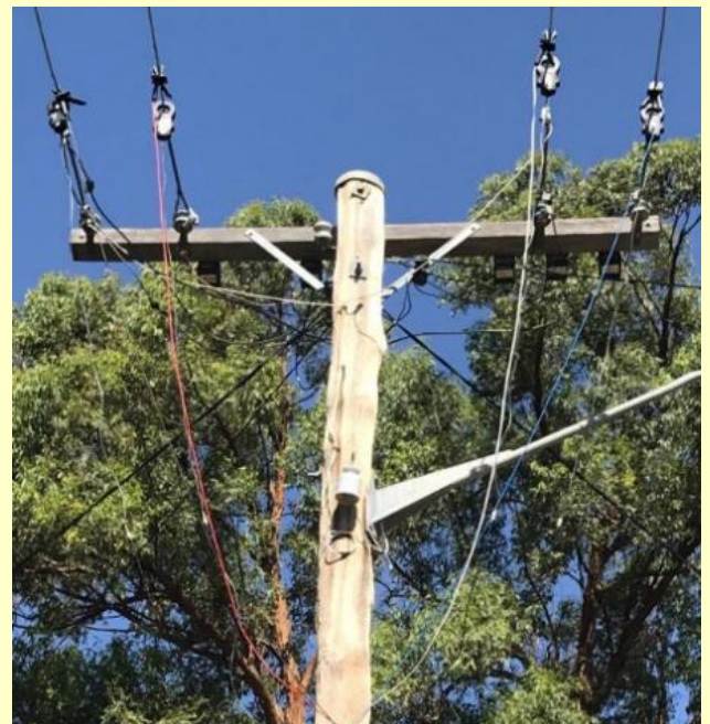
Figure 6: Current transformer probe and voltage clamps installed on overhead conductors
