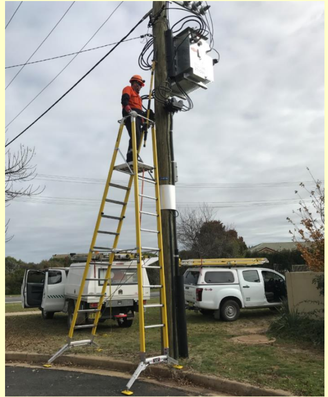
Figure 5: Current transformer probe and voltage clamp being installed, using hot stick and elevated work platform
