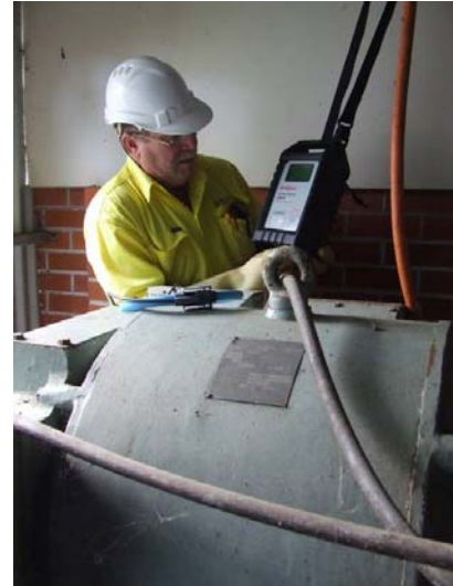
A PowerMonic 45, configured for voltage unbalance, is installed at a motor to determine the cause of overheating.
