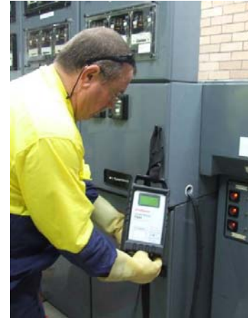
A PowerMonic 45 is installed on a transformer panel for temporary power quality monitoring.
