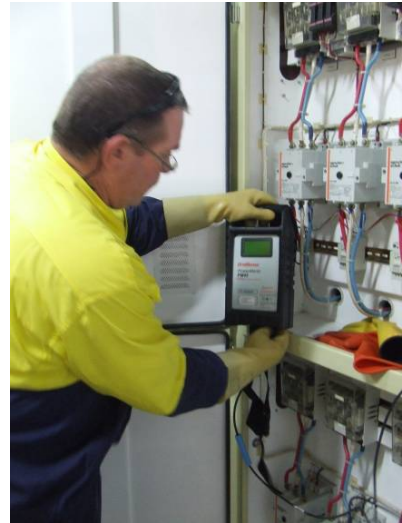
A PowerMonic 45 is installed at a plastics plant to determine cause of random shutdowns.
